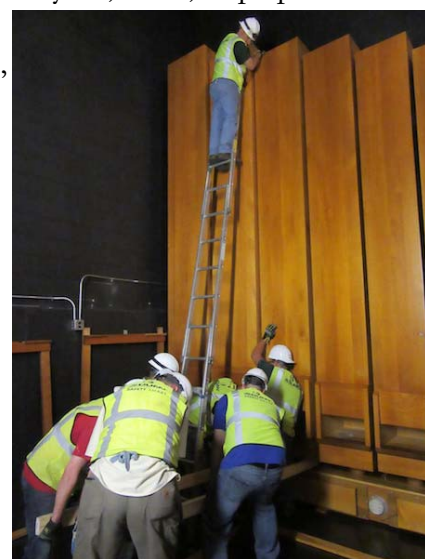
Foley-Baker crew installs basses of the 32' Pedal Bourdon in Northrop Auditorium. The largest pipe weighs 630 pounds.
